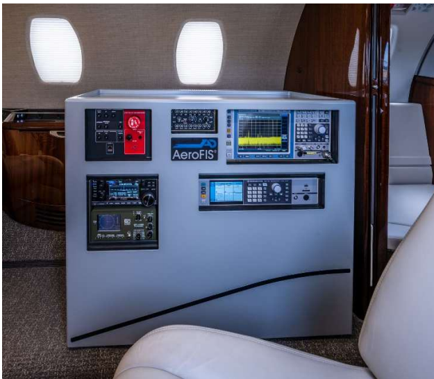
Figure 1: Example for a Modern AFIS Installation with a Digital Spectrum Analyzer (top right) and a Direction Finder (bottom left).
