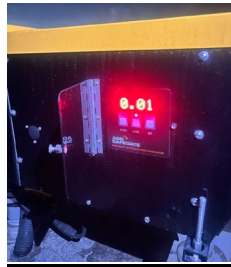
Built-in clinometer reading for PAPI Unit B (source: internal)
